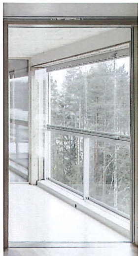
Glazed balconies as "Wintergarden" -frameless glass sliders
